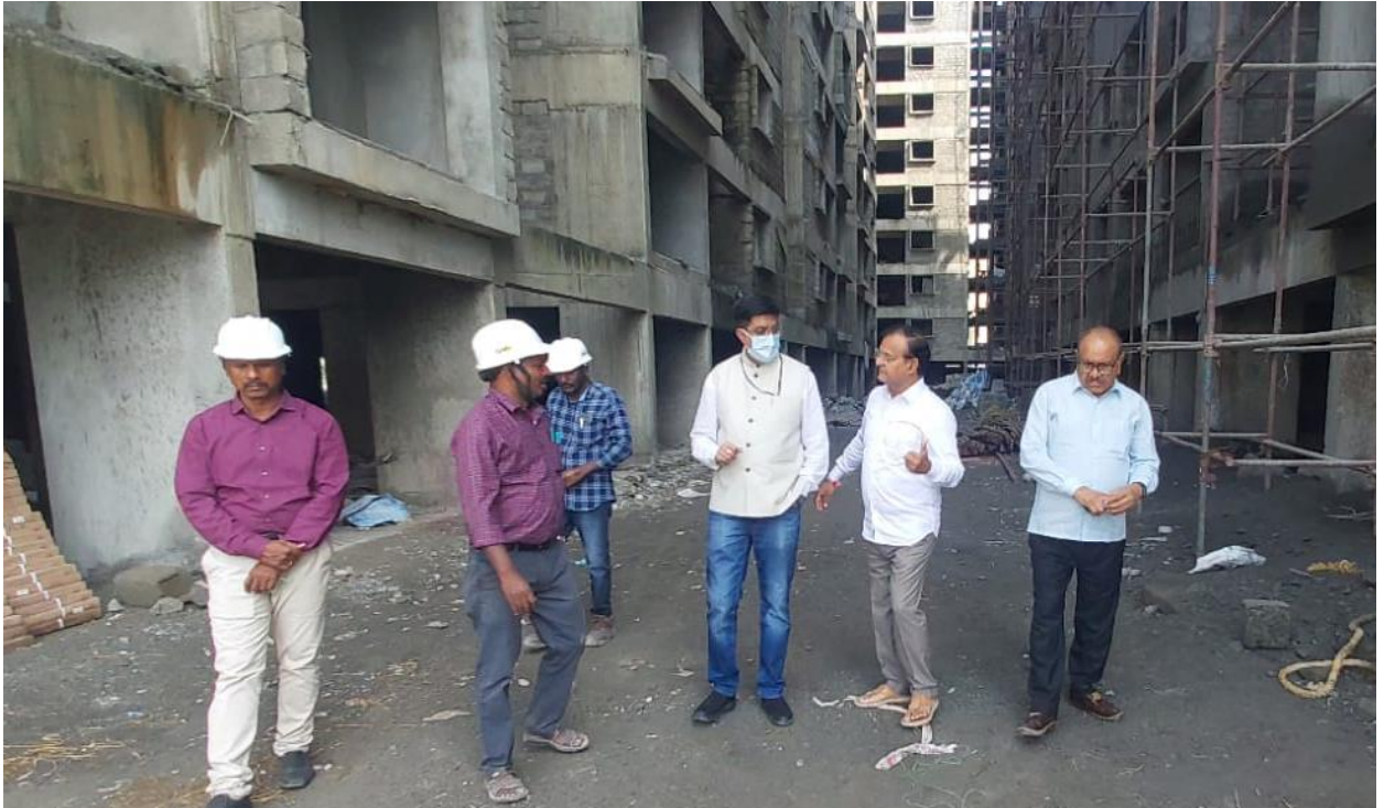
C.E.O & DIR(FIN), CGEWHO inspecting Construction activities along with M.D M/s SRICO Projects Pvt. Ltd.
